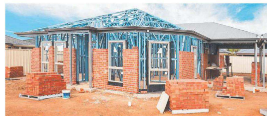
A slice of new stock needs to be set aside for low to moderate-income housing.
